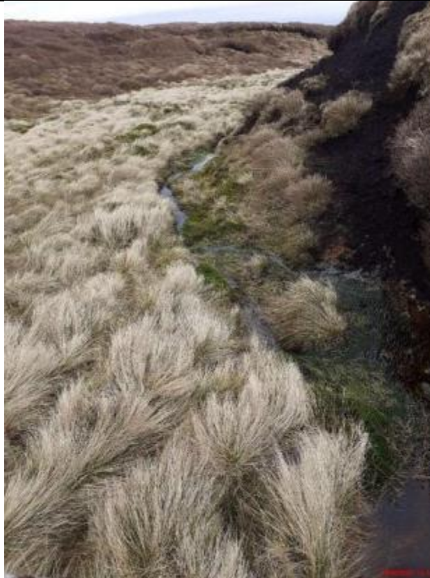
Photo 4 Photograph showing typical location for stone dam proposed for protection of re-profiled hagg edge/gully side at Twizle Head (Hagg edge/gully side shown prior to re-profiling).
